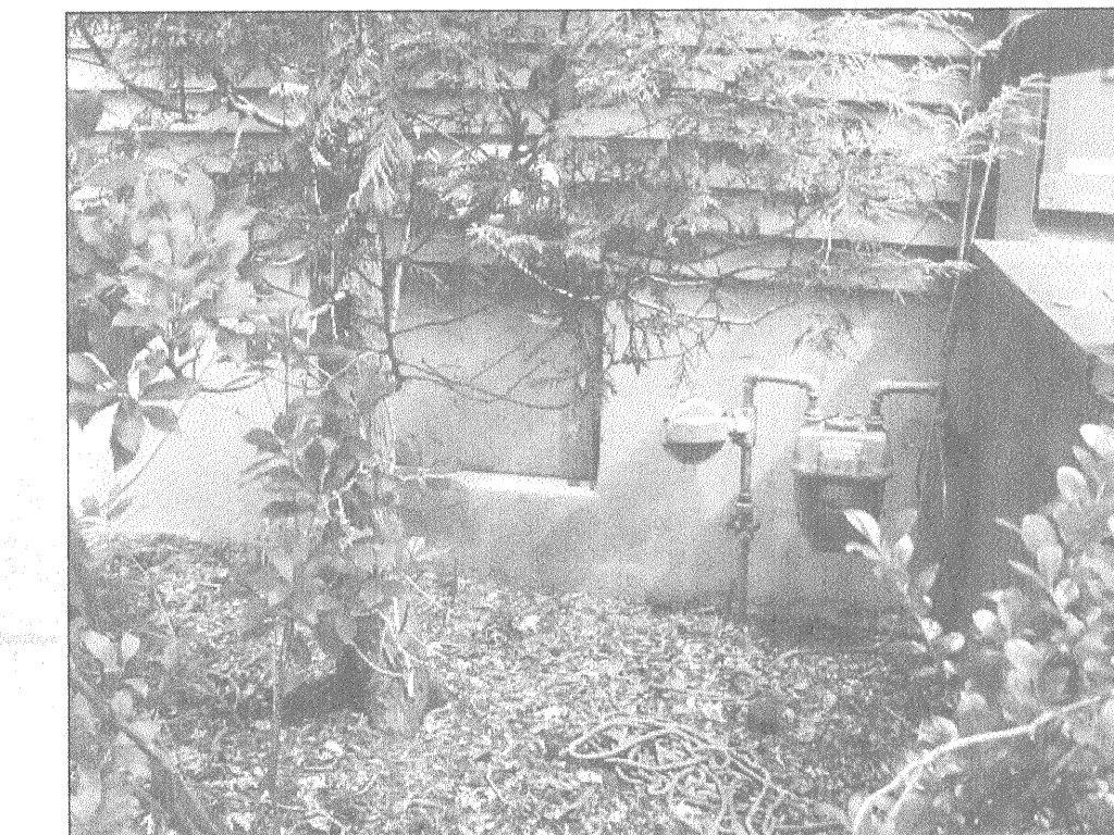
UTILITIES AT REAR
